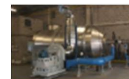
Wet & Dry Scrubbers
