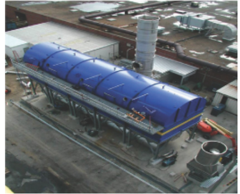
CECO Abatement Regenerative Thermal Oxidizer at a Chemical Plant
